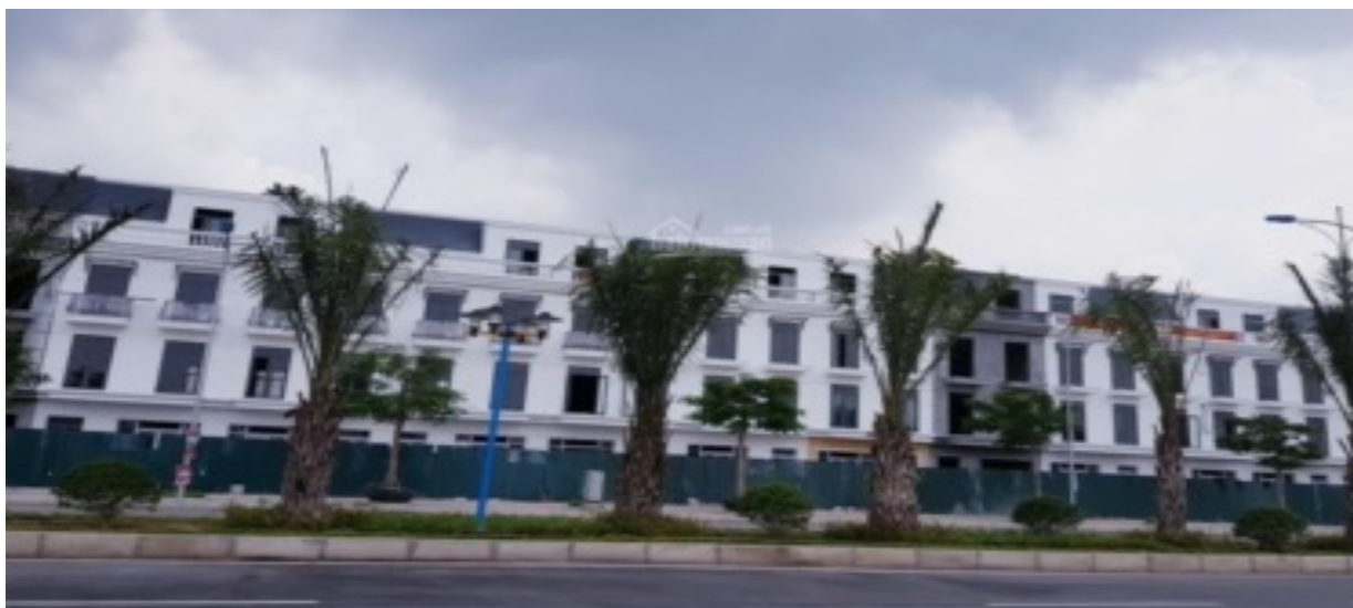
Trang Due Urban Area Hai Phong is deploying infrastructure and building commercial townhouses
